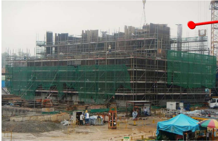
米埔通風樓之結構工程已大致完成 Structural construction for Mai Po Ventilation Building is substantially completed
