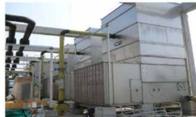
石崗大樓之冷卻水塔 Cooling Tower at Shek Kong Main Building
