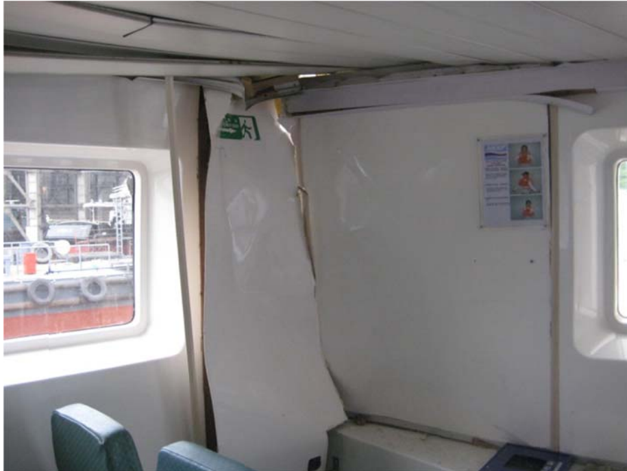
Figure 5: Photo showing the extent of damage to the part of Sea Smooth involved in the collision
