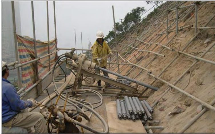
Use of soil nails to enhance the robustness of slope
