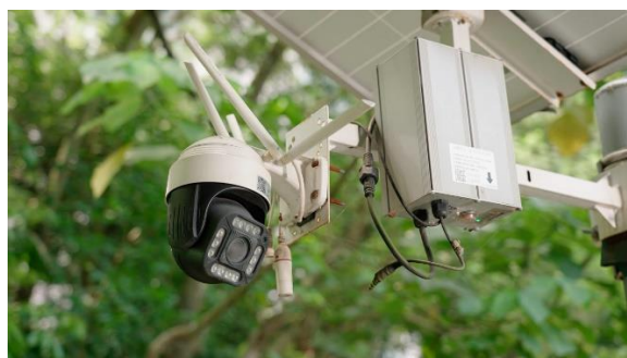
A monitoring system keeps real-time watch on the condition of stormwater outfalls to facilitate timely action.
