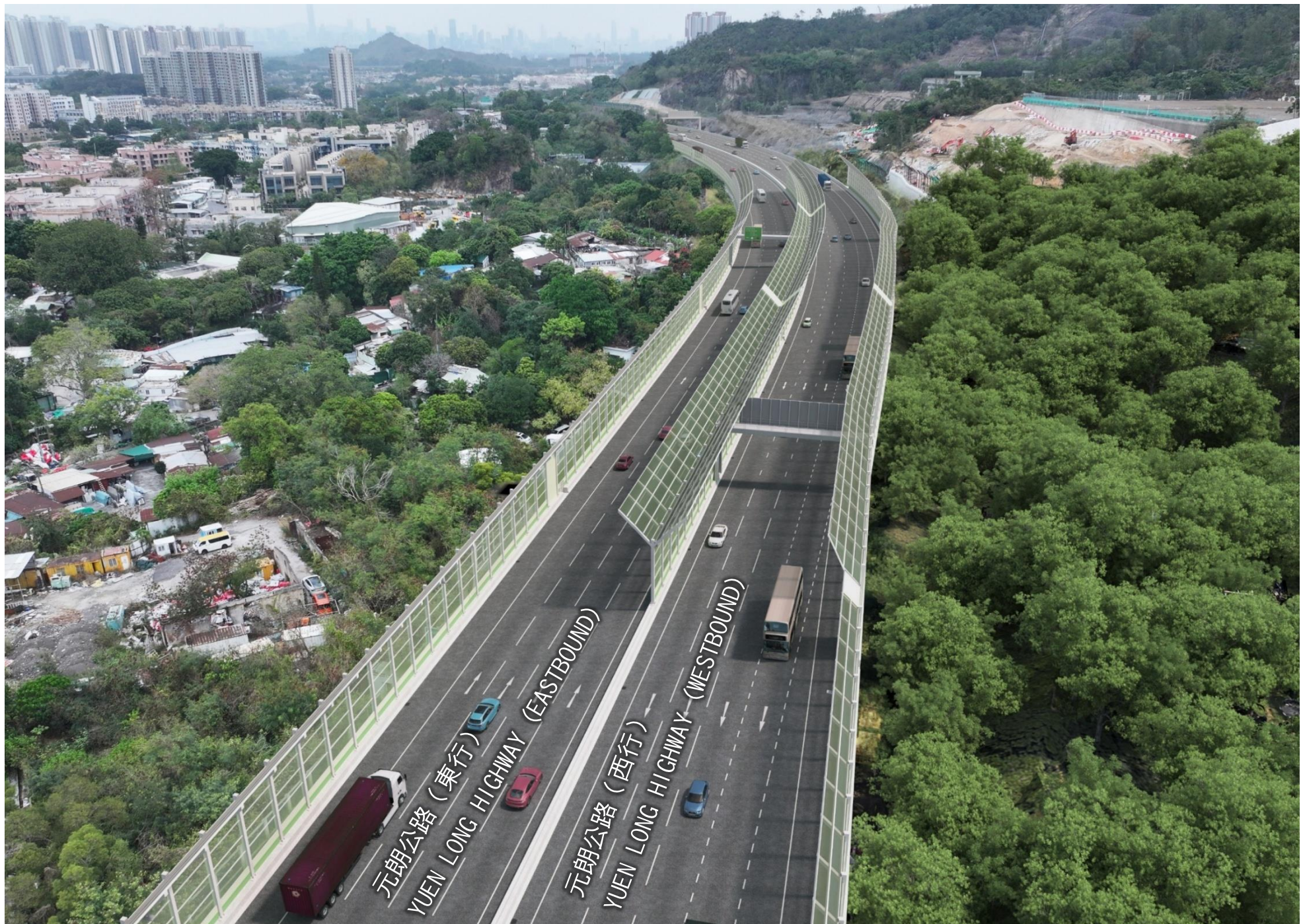
擴闊約 3 公里長的元朗公路為雙程四線分隔行車道 Widening of Yuen Long Highway (approximately 3-kilometre) to dual four-lane carriageway
